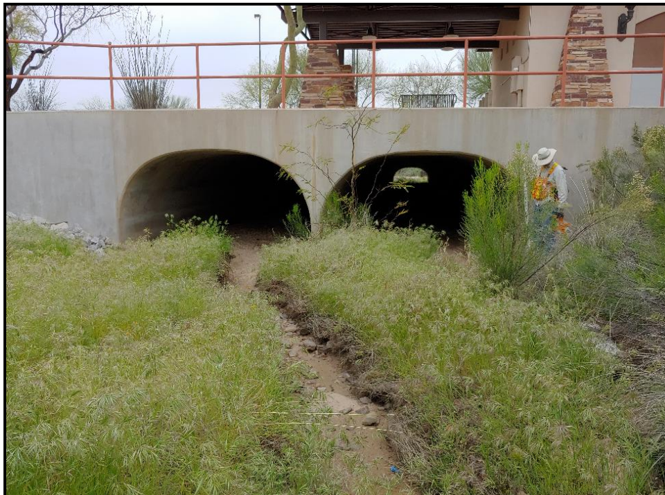
PHOTOGRAPH 19 Southern Culvert over Marketplace Access Road that Leads to Open Space and Big Wash
